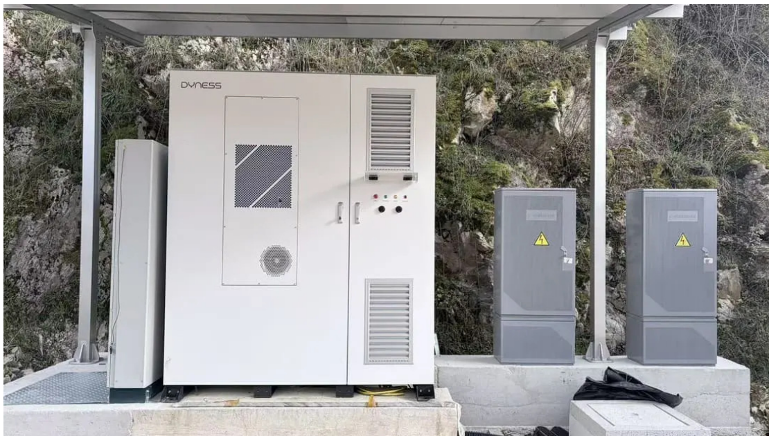
Dyness project photograph: DH200F, Italy.
