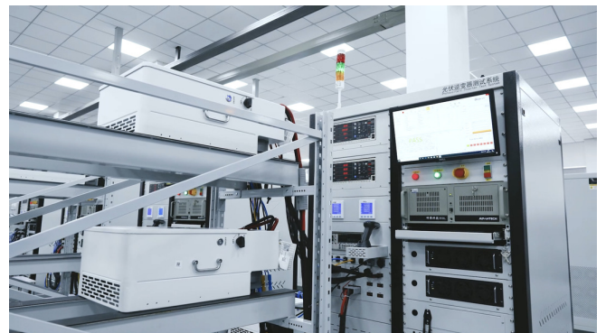
Deye inverter test system. Official image.
